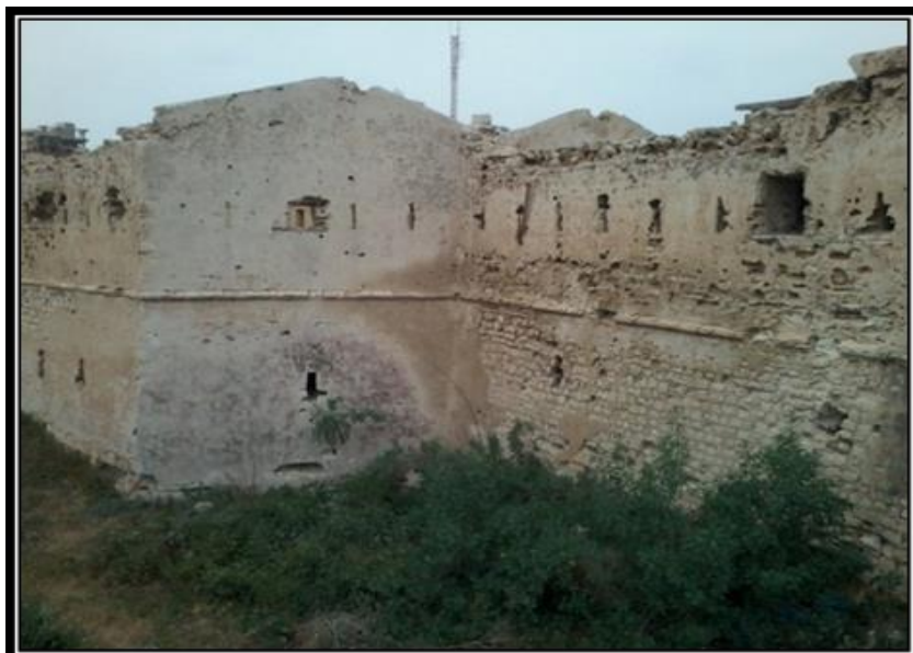
Figure 5: The effects of Moisture on the northern profile of the northern tower of Kousa Pasha Fort.
