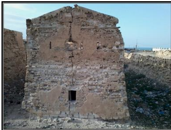
Figure 25: A vertical crack in the southern façade of the southern tower of Kousa Pasha Fort.
