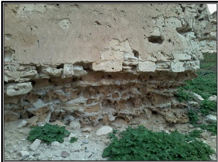
Figure 19: A model of lower erosion in the northern tower of Kousa Pasha Fort.
