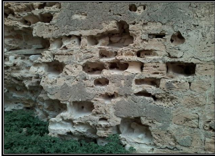
Figure 20: A model of the cavitation weathering on the southern tower of Kousa Pasha Fort.
