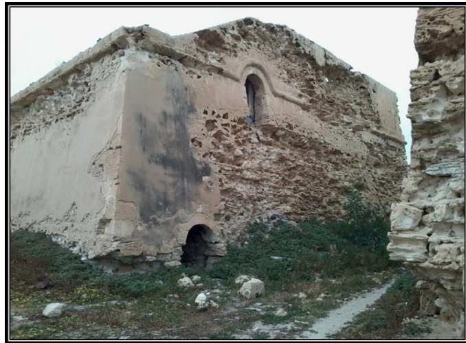
Figure 18: The effect of weathering processes in the Eastern façade of the southern tunnel of Kousa Pasha Fort.
