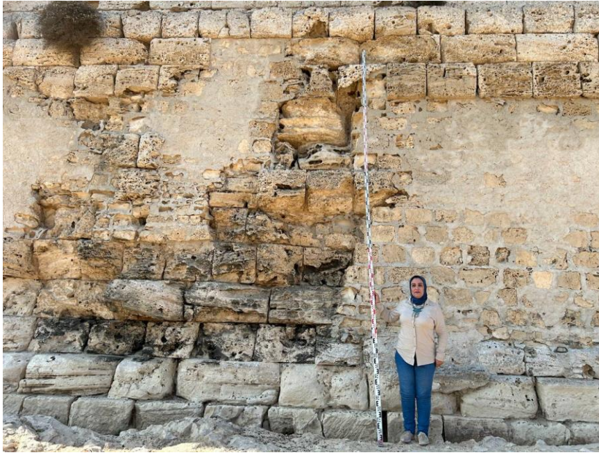
Fig. 6: Rainwater dissolution and weathering affect the limestone facade of the Taposiris Magna Temple.
